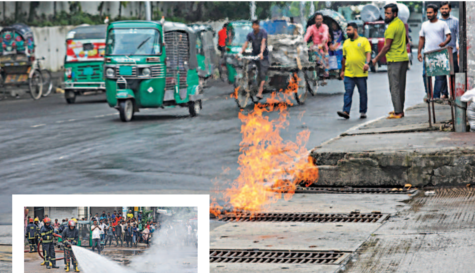
Flames shoot up from an underground gas pipeline after it burst on Zakir Hossain Road in the Foy's Lake area of Chattogram city yesterday afternoon, triggering panic among pedestrians and vehicle passengers. Fire service personnel brought the blaze under control after about an hour and a half of effort. PHOTO: STAR
