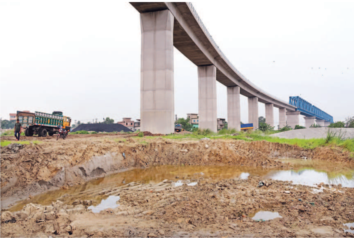
Large pits have emerged after soil was extracted from beneath the Padma rail link bridge in the Aliganj area of Narayanganj's Fatullah. The district administration yesterday halted the excavation following locals' concerns that the work could damage the structure. The photo was taken yesterday.
