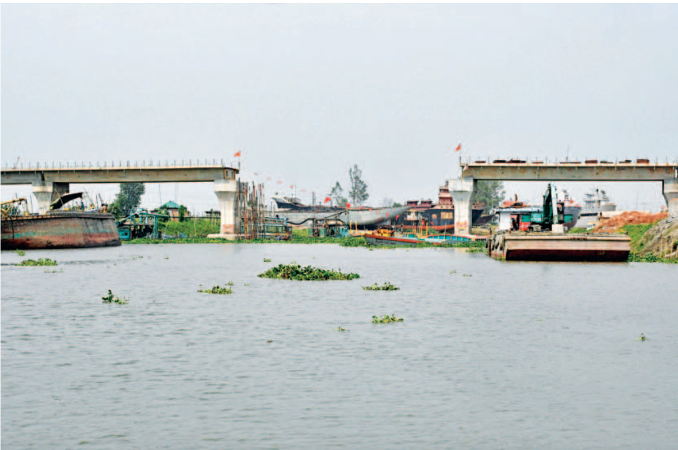
Eight years on, the construction work on the Mollarhat Bridge over a branch of the Dhaleshwari River in South Keraniganj remains unfinished, forcing thousands on both banks to rely on risky boats and makeshift crossings. The photo was taken recently.
