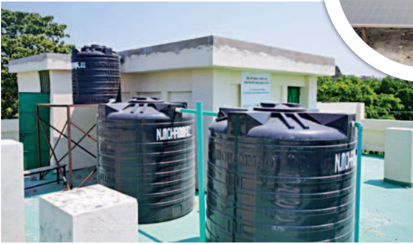
Rainwater harvesting tank at a school in Teknaf's Shilkhali village.
