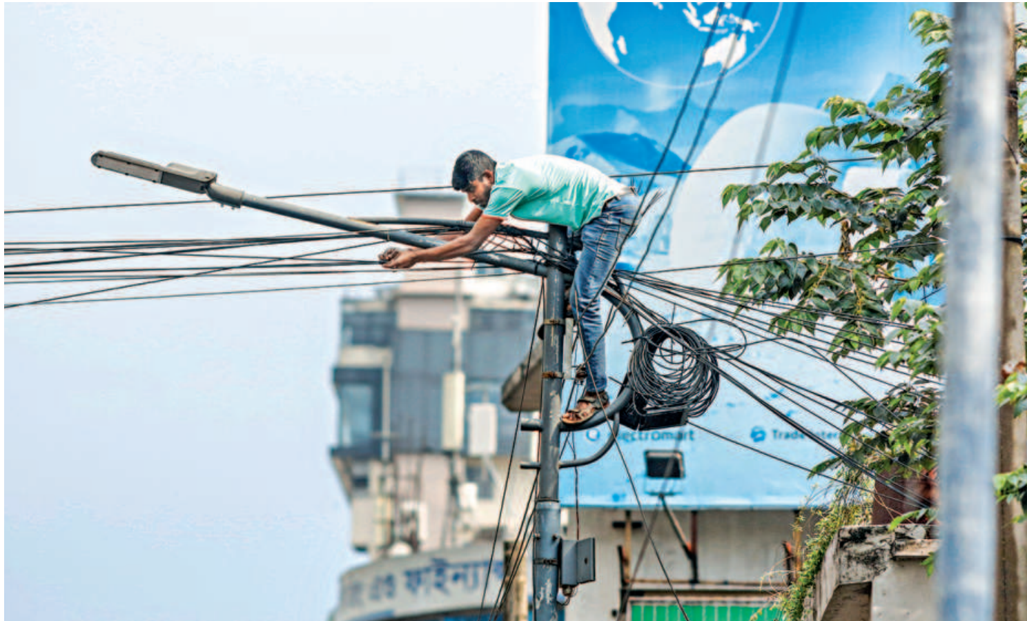
A worker perches precariously atop a light pole while carrying out maintenance work on internet cables in Dhaka's Banglamotor area yesterday. He appears to be working without any visible safety harness or protective gear amid a tangled web of overhead utility lines, risking serious injury.
