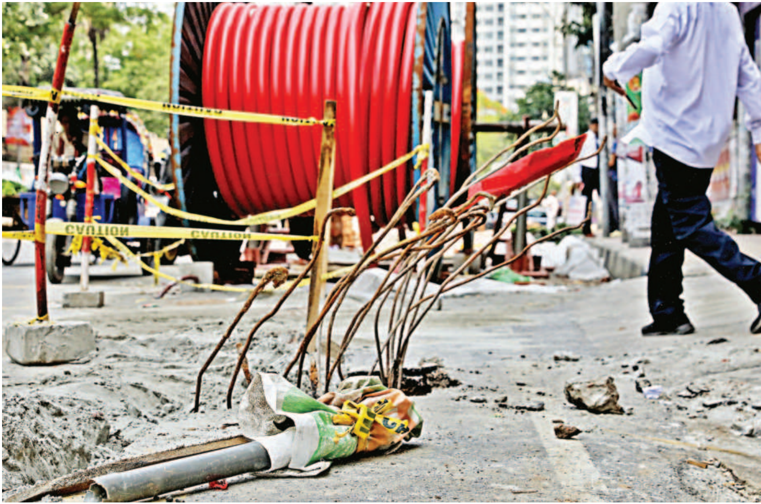
Rods protrude from a temporarily sand-filled section of a road in the capital's Segunbagicha area following underground cable installation work by the Dhaka Power Distribution Company. The absence of proper safety measures poses risks to pedestrians, especially at night. The photo was taken yesterday.
