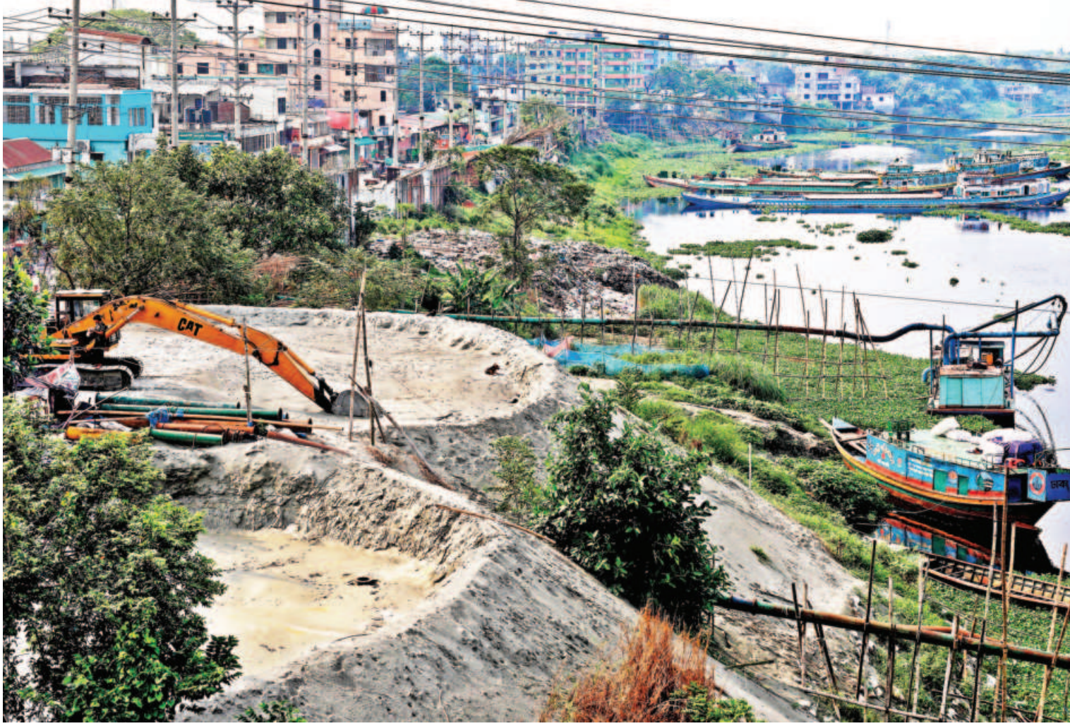
A local influential group is illegally trading sand after occupying a portion of the Bangshi river in the Nayarhat area of Savar, on the outskirts of Dhaka. The photo was taken recently.
