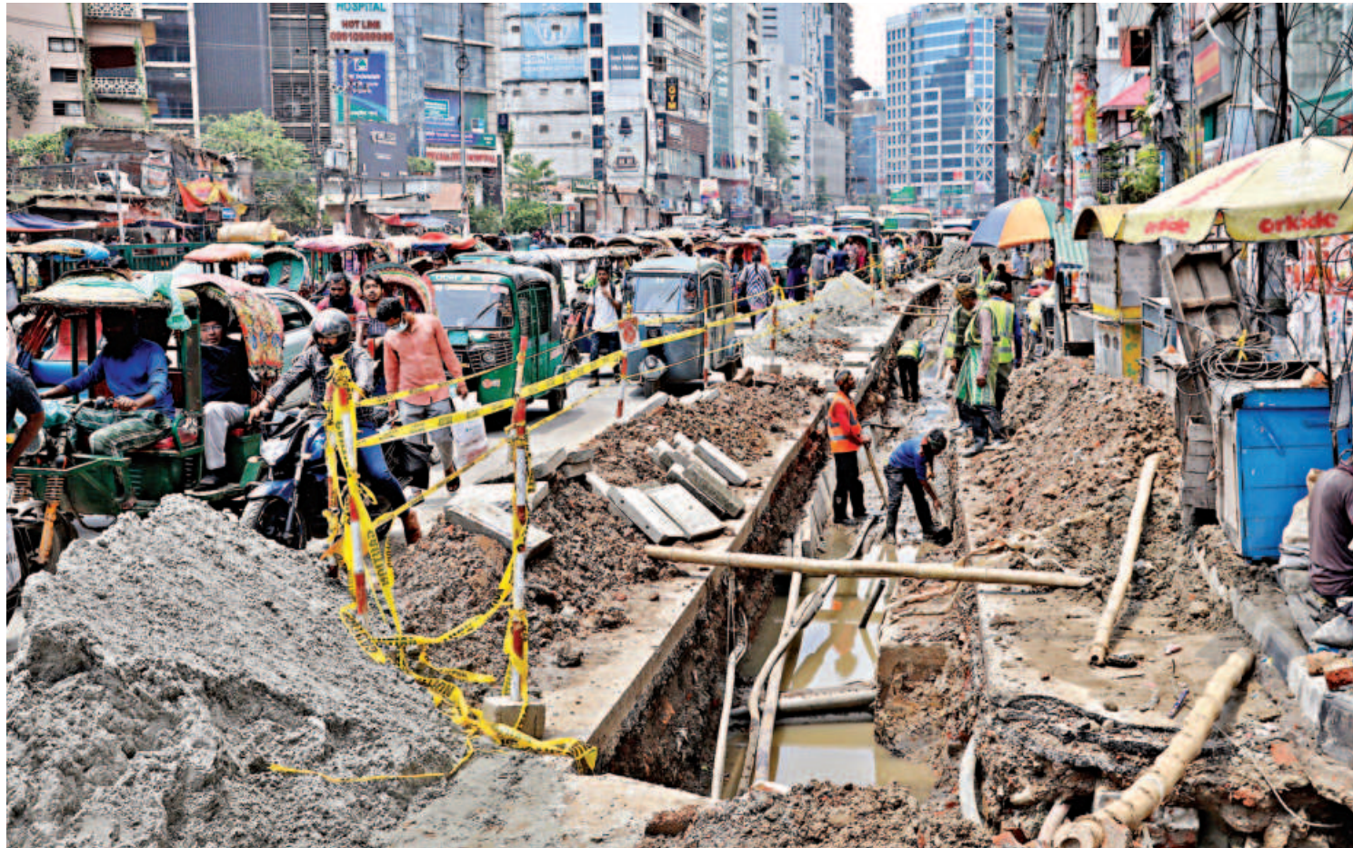
Commuters endure severe traffic congestion as underground cable installation work by the Dhaka Power Distribution Company Limited narrows the main road in the capital's Shantinagar area. The photo was taken yesterday.
