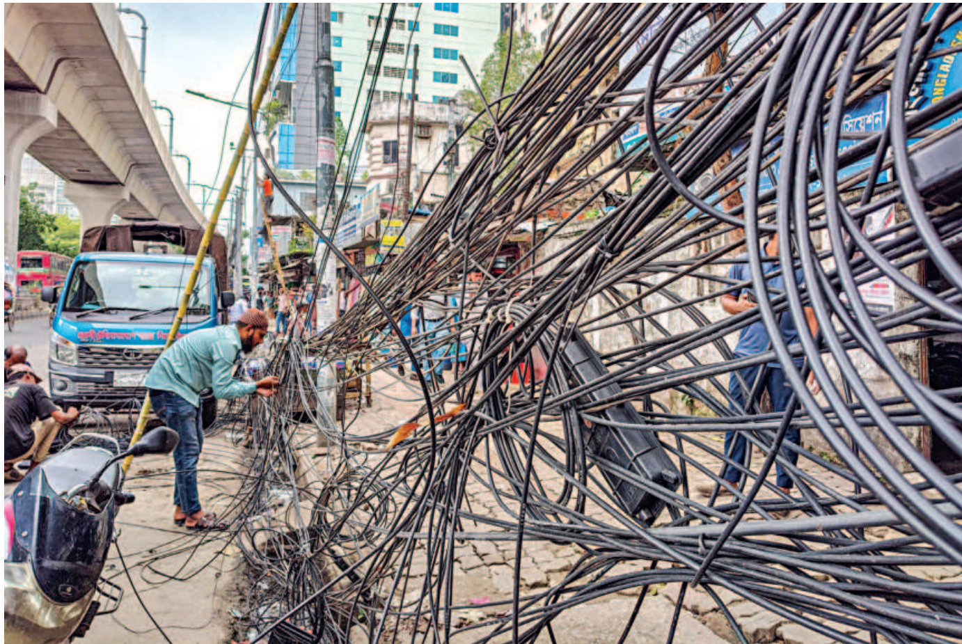
Workers reconnecting illegal fibre-optic cables to a utility pole on Topkhana Road in the capital's Purana Paltan just hours after authorities cleared hazardous overhead tangles to improve public safety and city aesthetics. Despite regular enforcement drives by city corporations, service providers often restore these connections immediately.
