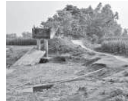
The bridge, over the Takimari canal on Alirpara-Gopalpur road, was washed away during the floods in 2019.
