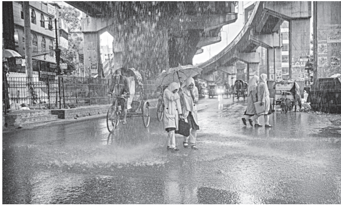
Rainwater cascades from the Muradpur-Lalkhan Bazar flyover in Chattogram during a recent downpour, as faulty drainage causes runoff to spill directly onto the road below, soaking pedestrians and disrupting traffic along the busy stretch.
