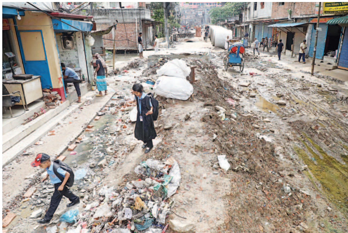
The sluggish pace of development work by Dhaka North City Corporation, including sewerage upgrades on Paris Road in the capital's Mirpur-11, continues to drag on, causing prolonged suffering to everyday commuters, especially schoolchildren and office-goers. The photo was taken recently.
