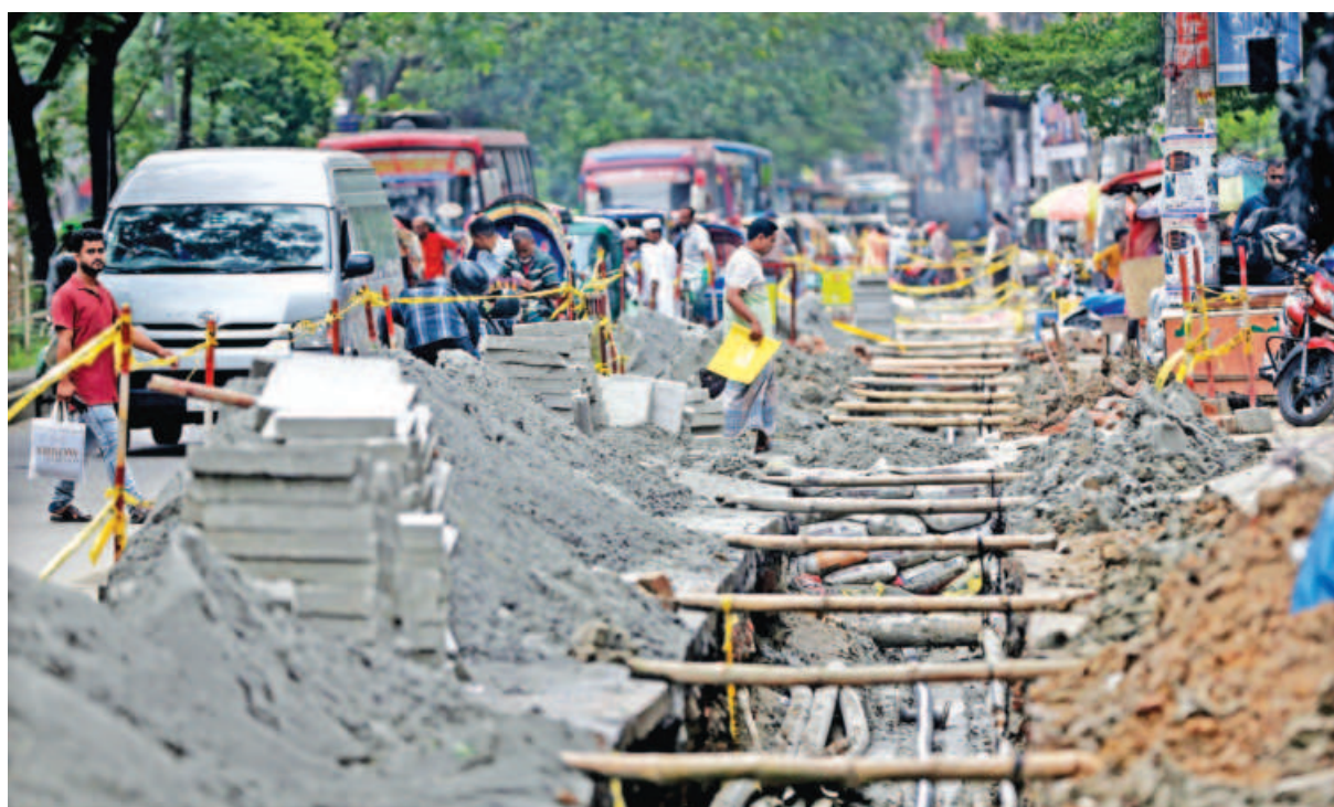
Dhaka Power Distribution Company is installing underground power lines in the capital's Bijoy Nagar area, but the work is progressing slowly, leading to increased traffic congestion and growing public suffering. PHOTO: FIROZ AHMED
