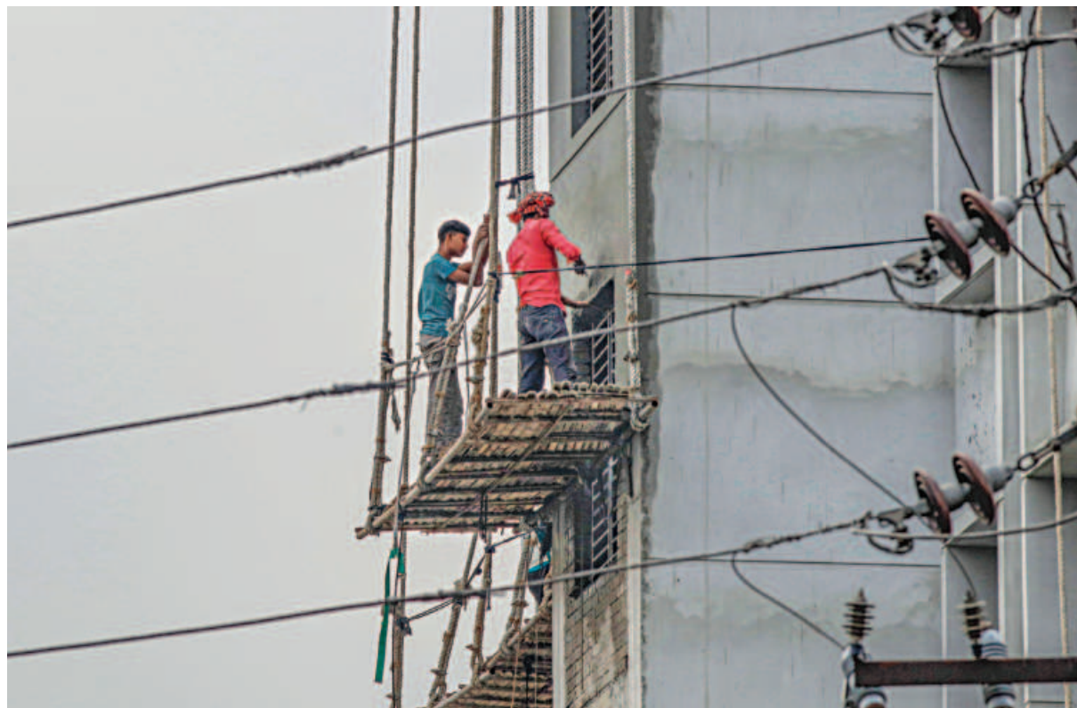
On a suspended bamboo scaffold six floors above the ground, two construction workers plaster the side of a high-rise government building. Without any safety harnesses or protective gear, the risk of a fall is serious. The photo was taken yesterday near the capital's Tejgaon Truck Stand area. PHOTO: RASHED SHUMON
