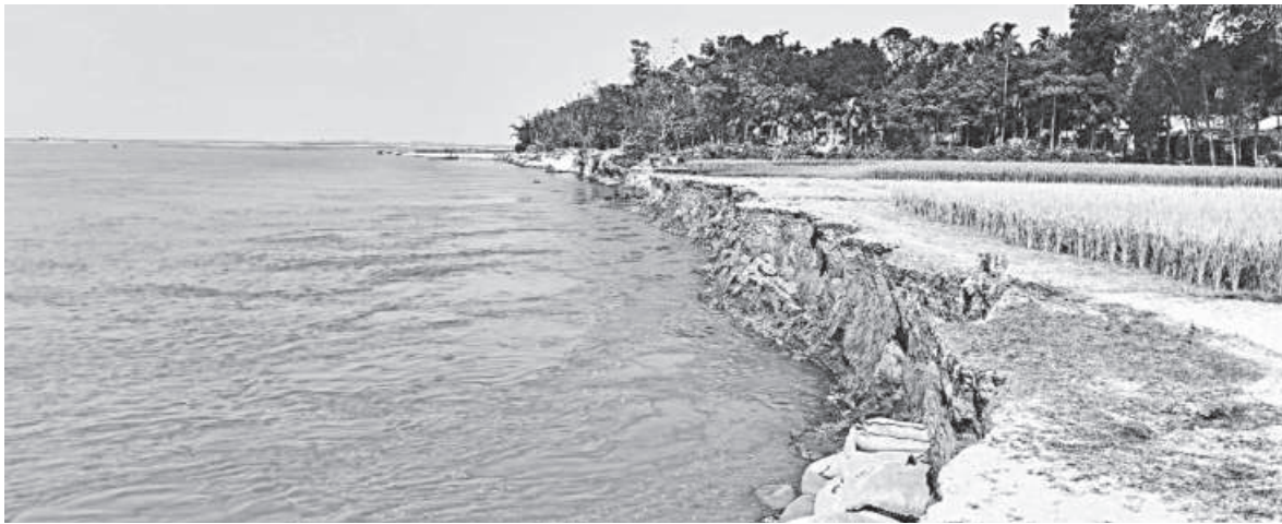
The latest erosion has intensified in Char Shoulmari union, particularly in Char Gendar Alga, Sonapur, West Khedaimari, Sukhurbati, Ghughumari, and Namazer Char. The photo was taken recently.
