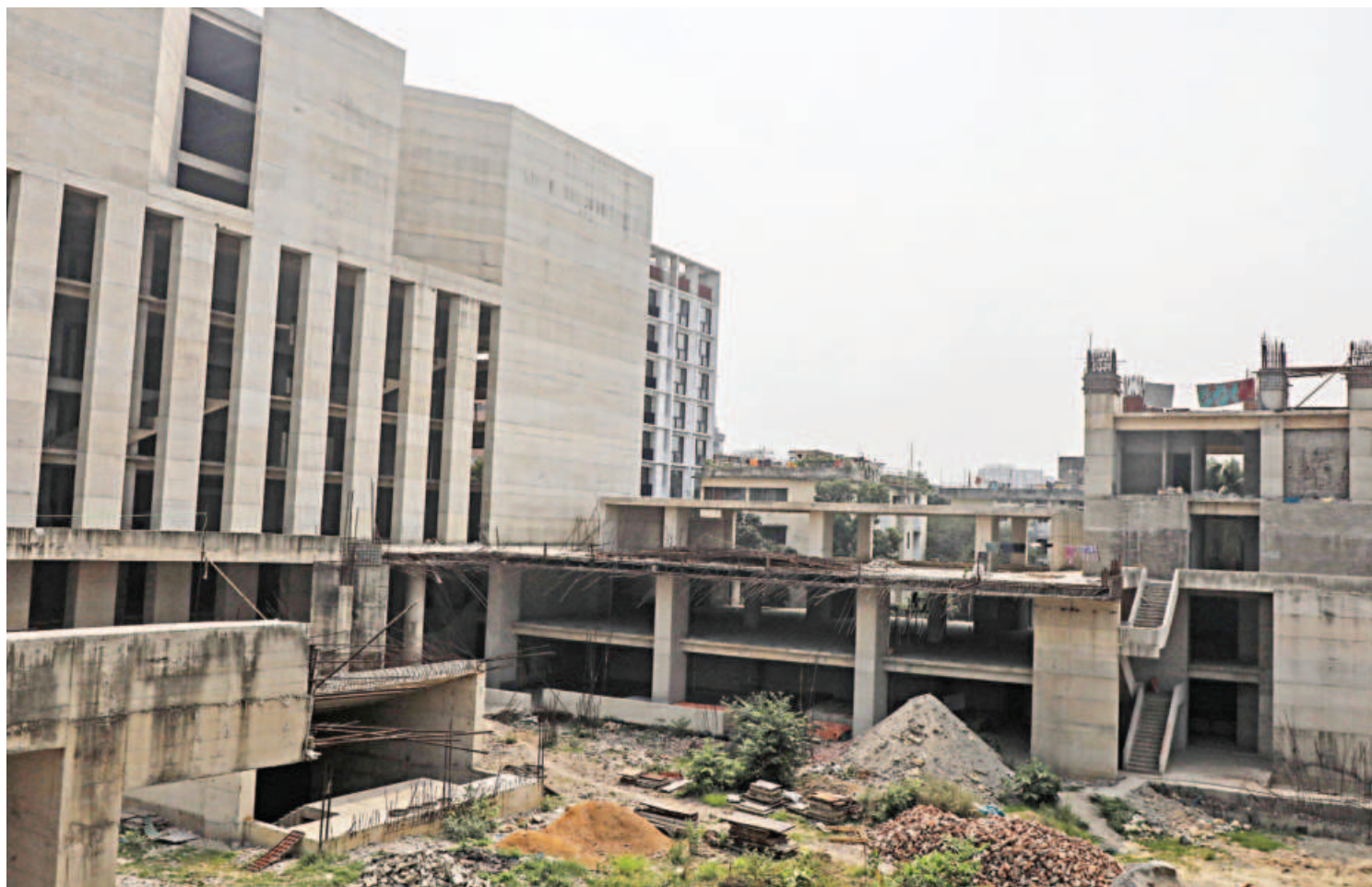
The project to modernise Sofia Kamal National Public Library, originally scheduled for completion in December 2024, saw significant delays stemming from design-related complications. The photo was taken yesterday.
