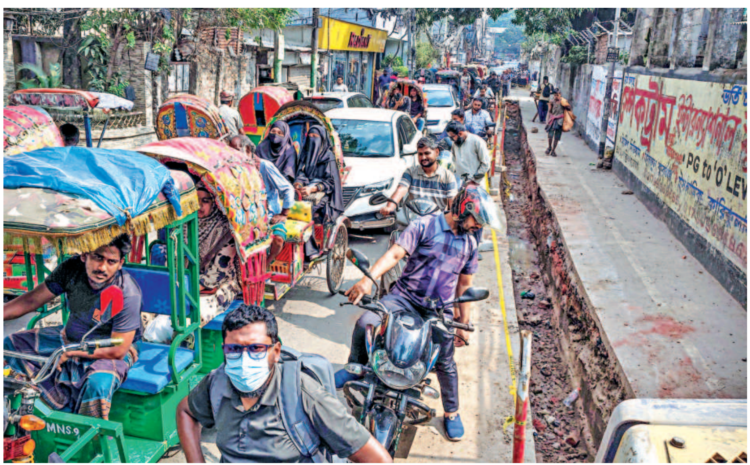
People stuck in traffic under scorching heat on a narrow street in Segunbagicha in Dhaka yesterday. Bikers occupy one lane while queuing for a nearby petrol pump, and roadwork by Dhaka South City Corporation has excavated another, leaving little space for commuters. PHOTO: RASHED SHUMON
