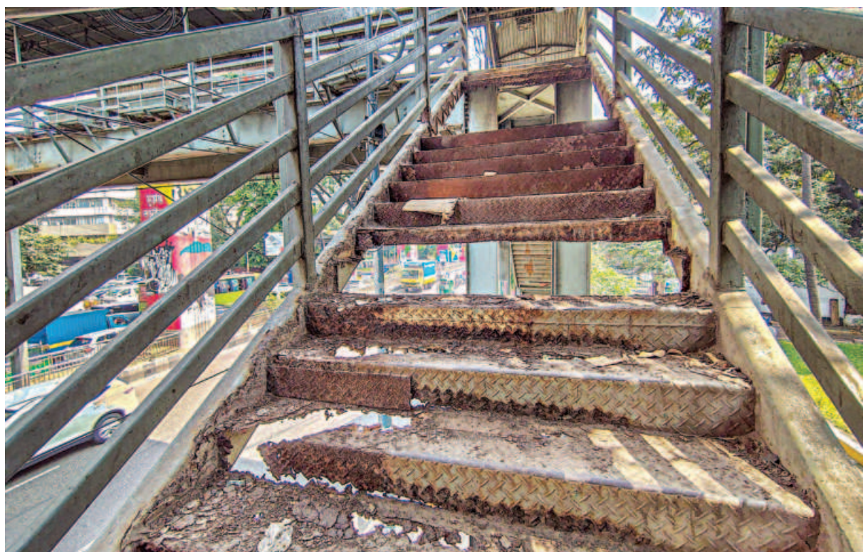
A dilapidated footbridge on Kazi Nazrul Islam Avenue near Paribagh in the capital. It has remained unusable for pedestrians for months.
