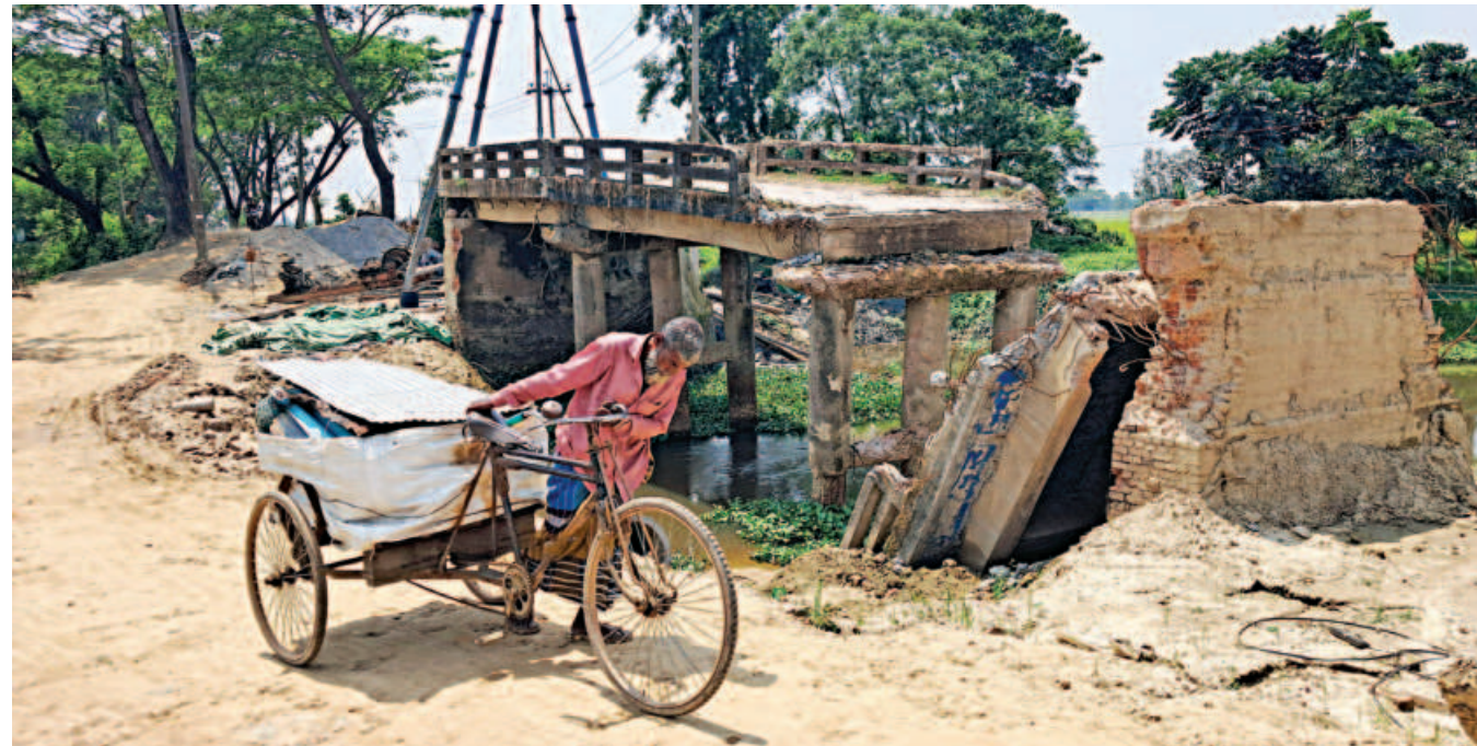
A man pushes a loaded cycle van past the collapsed bridge over the Kakina canal in Brahmanbaria's Moniando area, which has remained out of service for over a year. Slow reconstruction has kept direct road communication between Kasba and Akhaura upazilas suspended, forcing locals to rely on an earthen alternative route and endure prolonged hardship. PHOTO: MASUK HRIDOY
