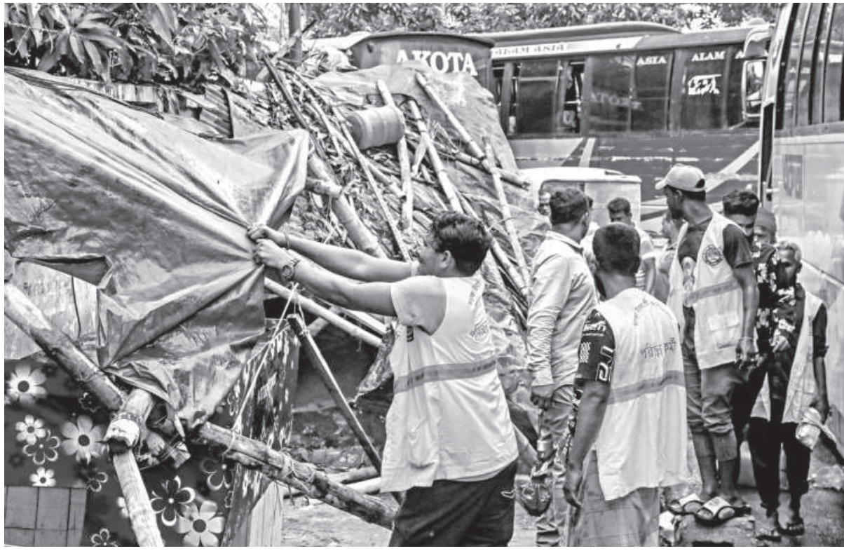
Dhaka City Corporation authorities conduct a drive at the Gabtoli bus terminal area in Dhaka to remove illegal structures and unauthorised vendors. The photo was taken yesterday.
