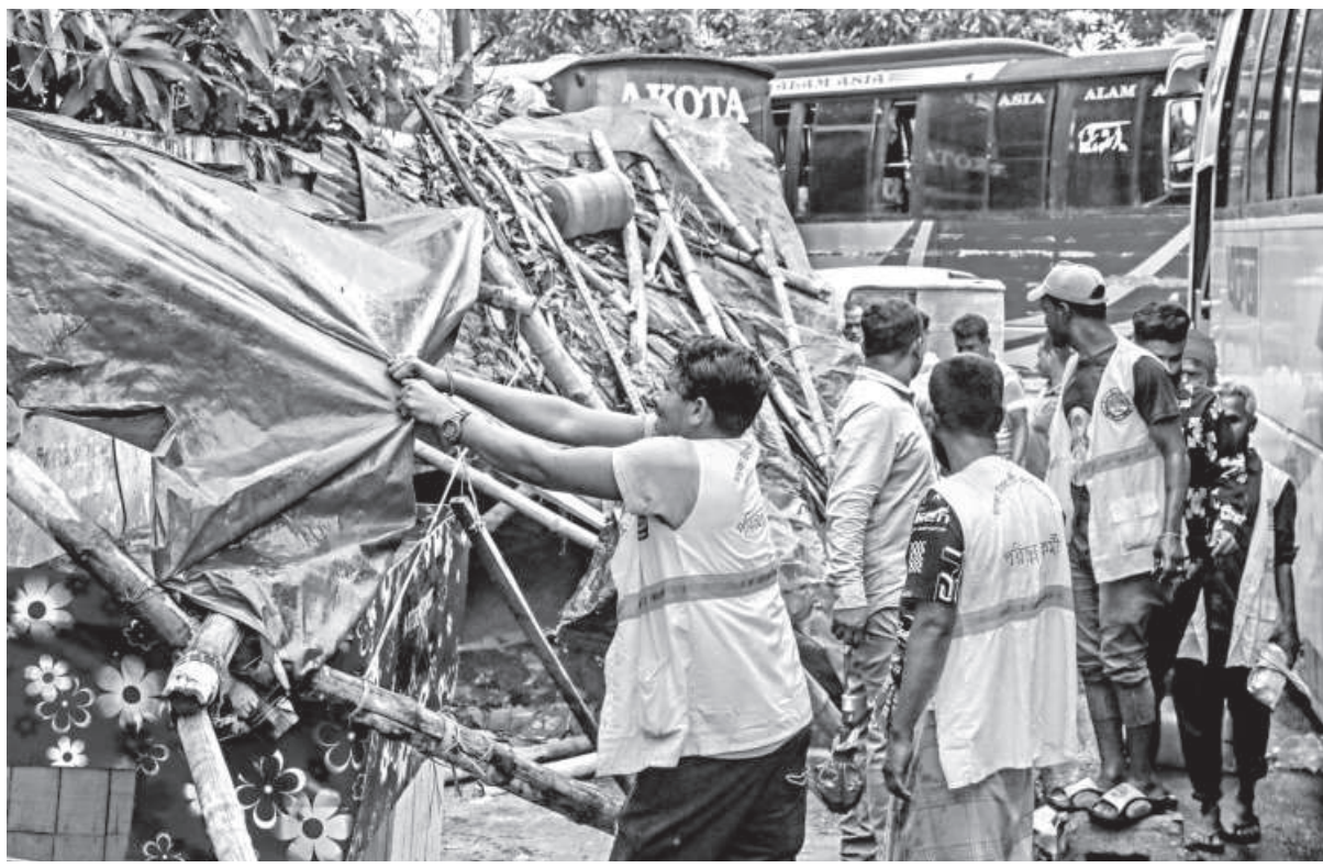
Dhaka City Corporation authorities conduct a drive at the Gabtoli bus terminal area in Dhaka to remove illegal structures and unauthorised vendors. The photo was taken yesterday.
