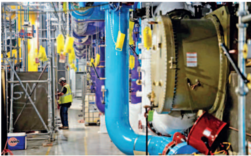
A person works inside the Microsoft data centre campus' graphical processing unit in Mount Pleasant, Wisconsin. PHOTO: REUTERS/FILE
