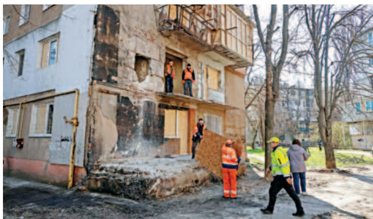
Workers install OSB boards in the places of broken windows at the site of an apartment building hit by a Russian drone strike in Odesa, Ukraine, yesterday.
