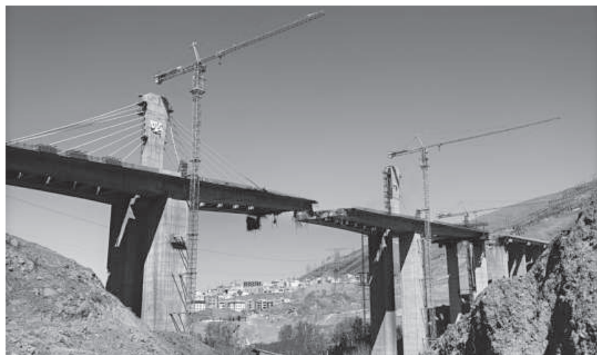
The B1 bridge damaged by a strike, as the US-Israeli conflict with Iran continues, in Karaj, Iran, yesterday.
