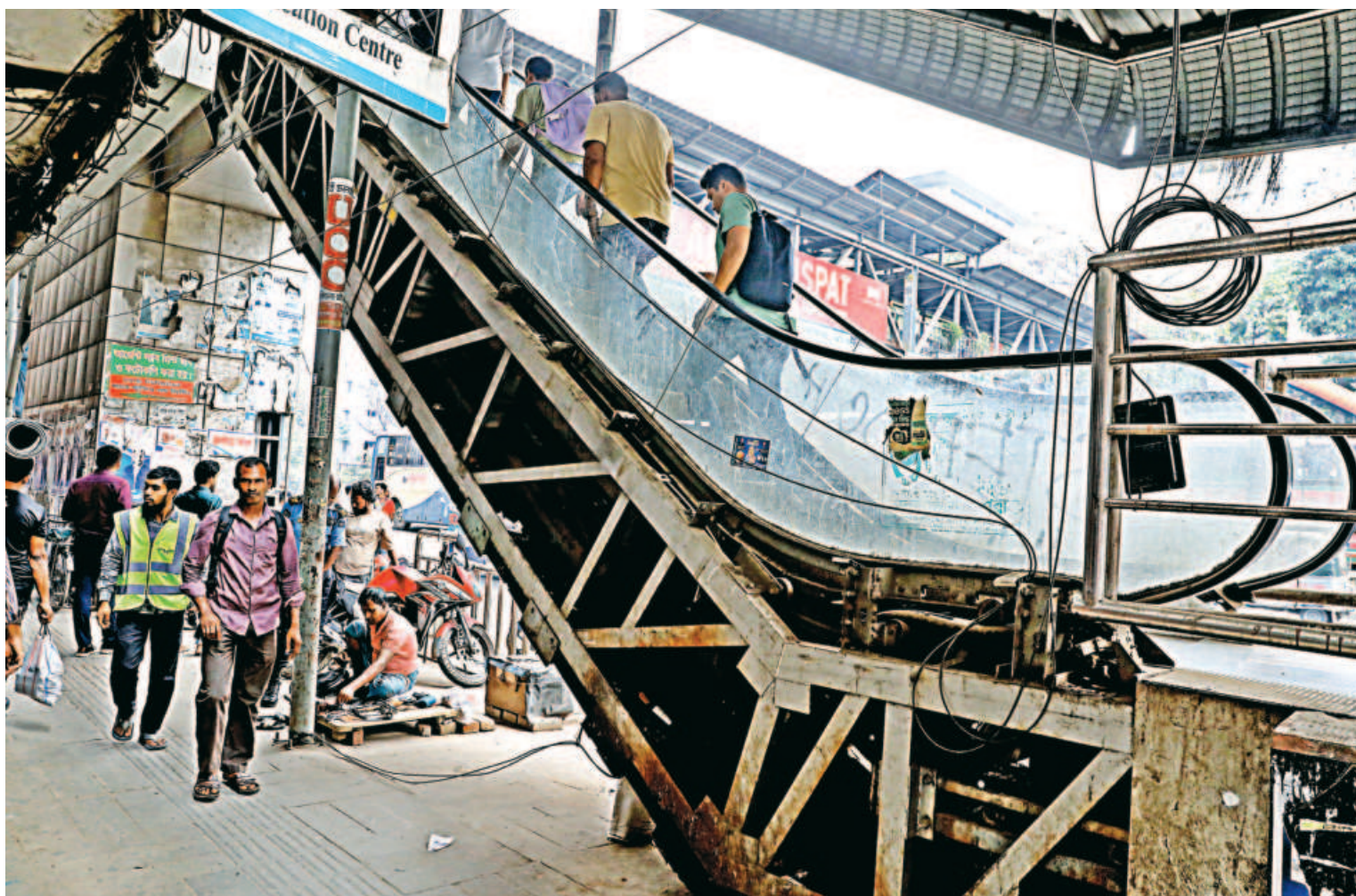
The escalator linked to a footbridge in Banani, Dhaka lies out of service, covered in rust, grease and dirt. Meant to aid the elderly, injured and persons with disabilities, its failure now limits safe road crossing. The photo was taken recently.
