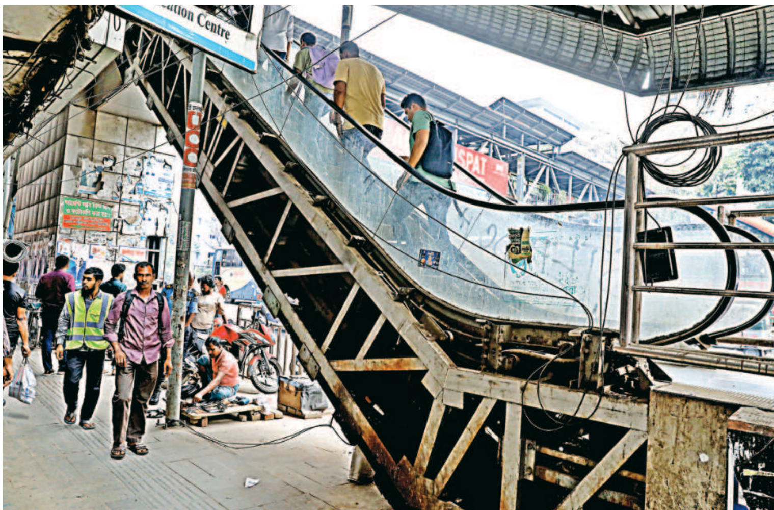
The escalator linked to a footbridge at Banani in Dhaka lies out of service, covered in rust, grease and dirt. Meant to aid the elderly, injured and persons with disabilities, its failure now limits safe road crossing. The photo was taken recently.
