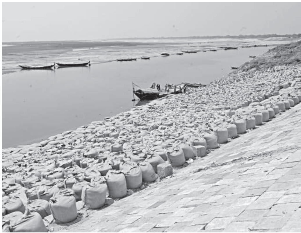
Sandbars have emerged across much of the western bank of the Padma River in the Aibadh area of Rajshahi city, making it appear fragmented into narrow canals. Boat movement has come to a halt, while the Water Development Board has begun work beneath the city protection embankment ahead of the monsoon. The photo was taken recently.
