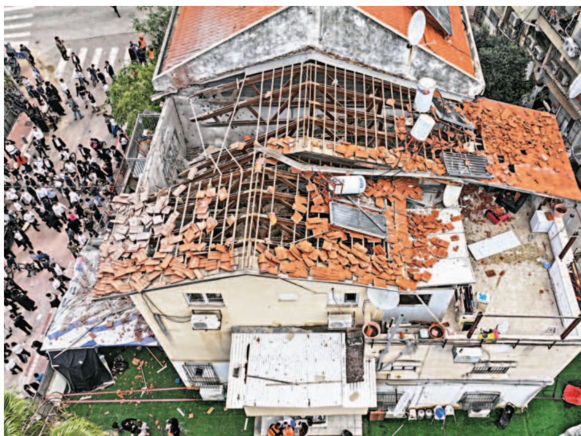
Drone view shows people gathering at a damaged residential area in Bnei Brak, central Israel, after Iranian missile barrages yesterday.
