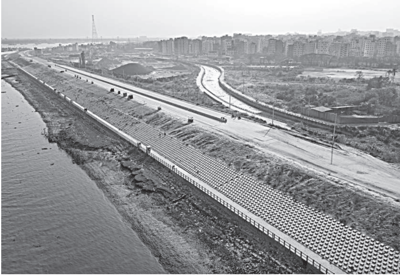
Work on the Kalurghat-Chaktai road and dyke project in Chattogram is still underway, nearly nine years after it was launched in July 2017 with a completion target of three years.
