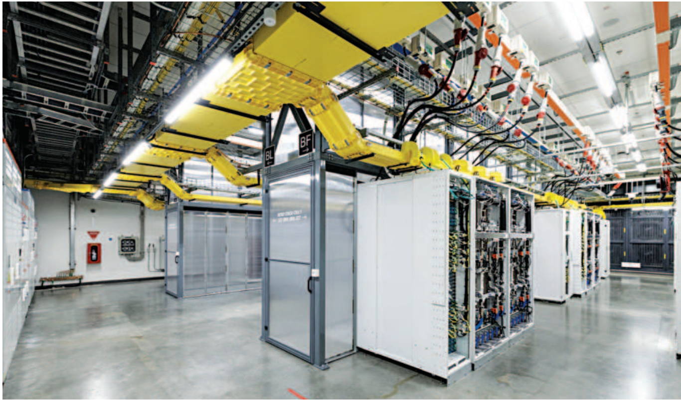
In this photo, racks of graphics processing units with a closed-loop liquid cooling system are seen inside an operational Microsoft data centre in Karawang, West Java.
