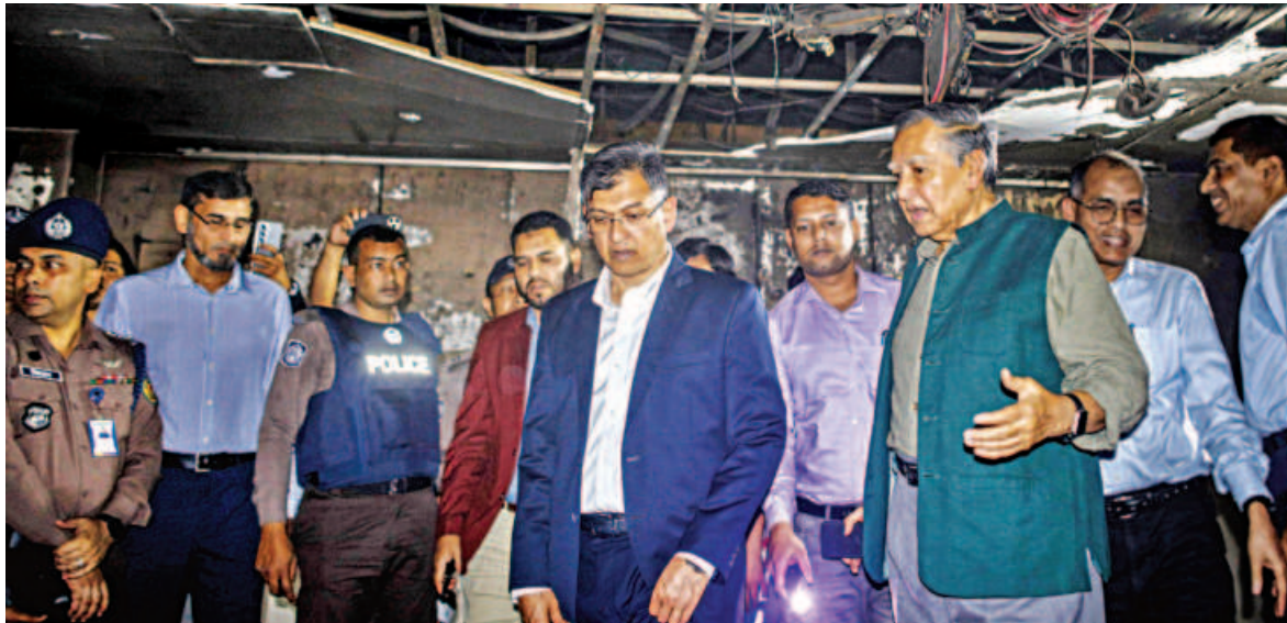
Home Minister Salahuddin Ahmed, accompanied by The Daily Star Editor and Publisher Mahfuz Anam, inspects the fire-damaged floors of the newspaper's building during a visit yesterday. Foreign Minister Khalilur Rahman also visited The Daily Star yesterday.
