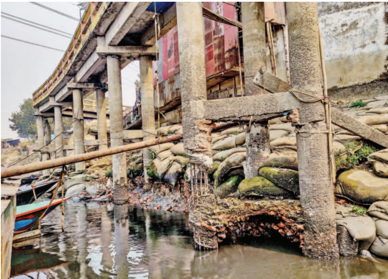
The pillars of a walkway on the bank of the Turag river in Gabtoli, Dhaka, have eroded, exposing the iron rods inside. The structure risks collapse unless urgent repairs are carried out. Aggravating the damage, boats are illegally anchored to the weakened pillars. The photo was taken yesterday.
