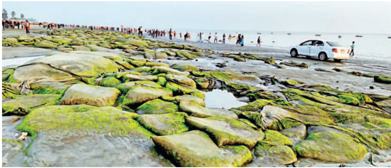
Around five- to six-year-old sand-filled geo-bags lie along Kuakata Sea Beach, with algae growing on them over time. Although installed to prevent beach erosion, the geo-bags have become hazardous as algae and dents make them slippery and unsafe for locals and tourists. The photo was taken recently.
