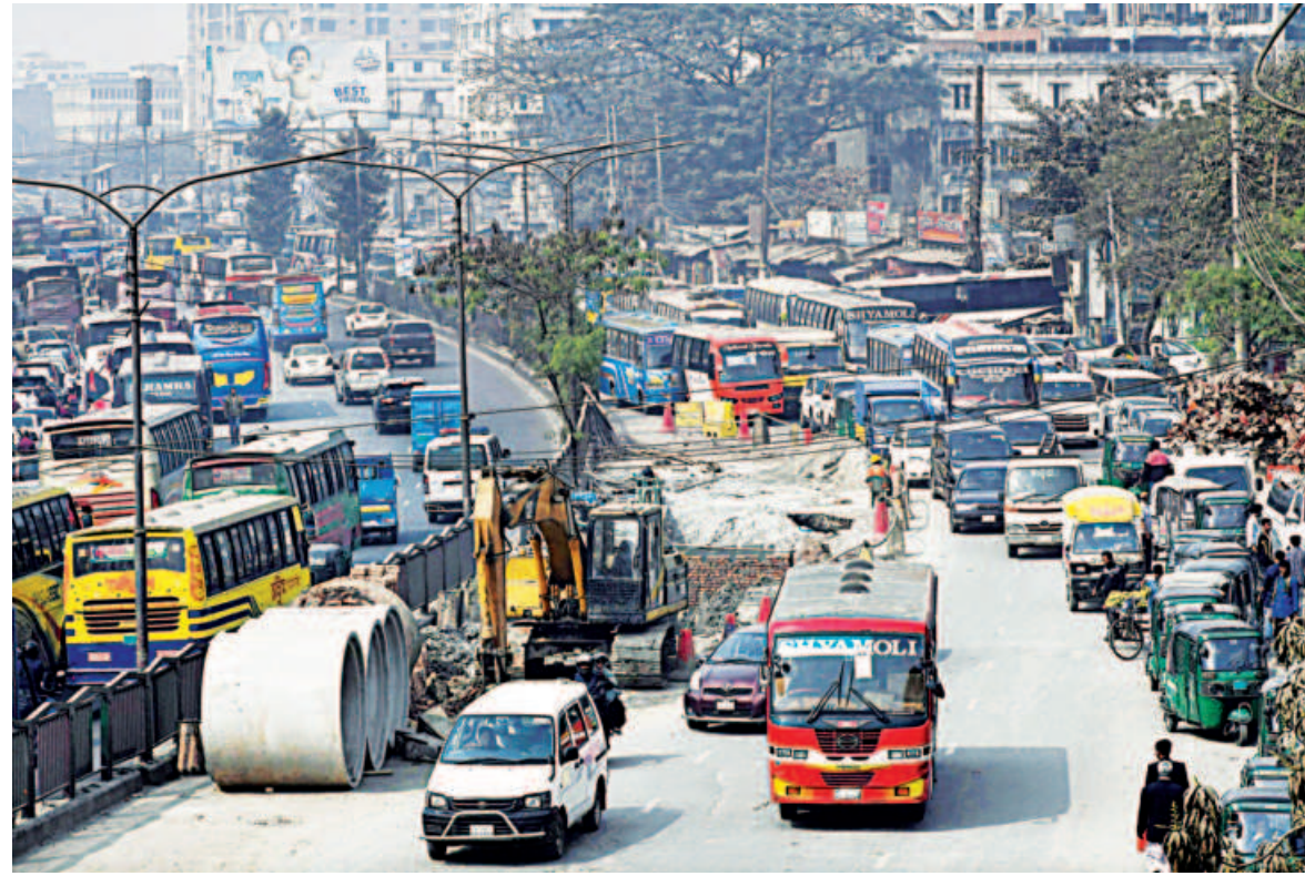
Dhaka North City Corporation is digging up part of the lane leading from Gabtoli to Technical to install sewage pipes. The work, which occupies half of this busy entry point to the capital, leaves vehicles stuck for long periods. The photo was taken yesterday.
