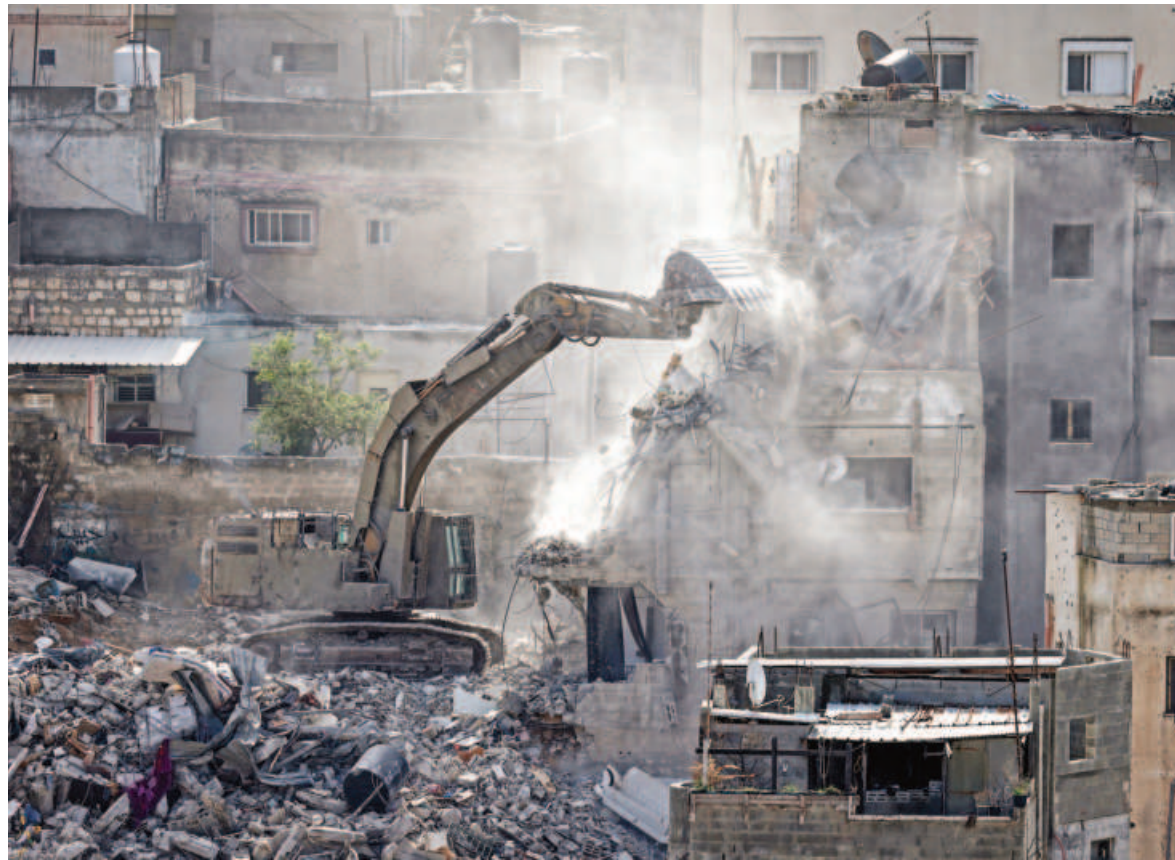
An Israeli military excavator demolishes one of 25 residential buildings earmarked for removal in the Nur Shams refugee camp, east of Tulkarem in the northern Israeli-occupied West Bank yesterday. PHOTO: AFP
