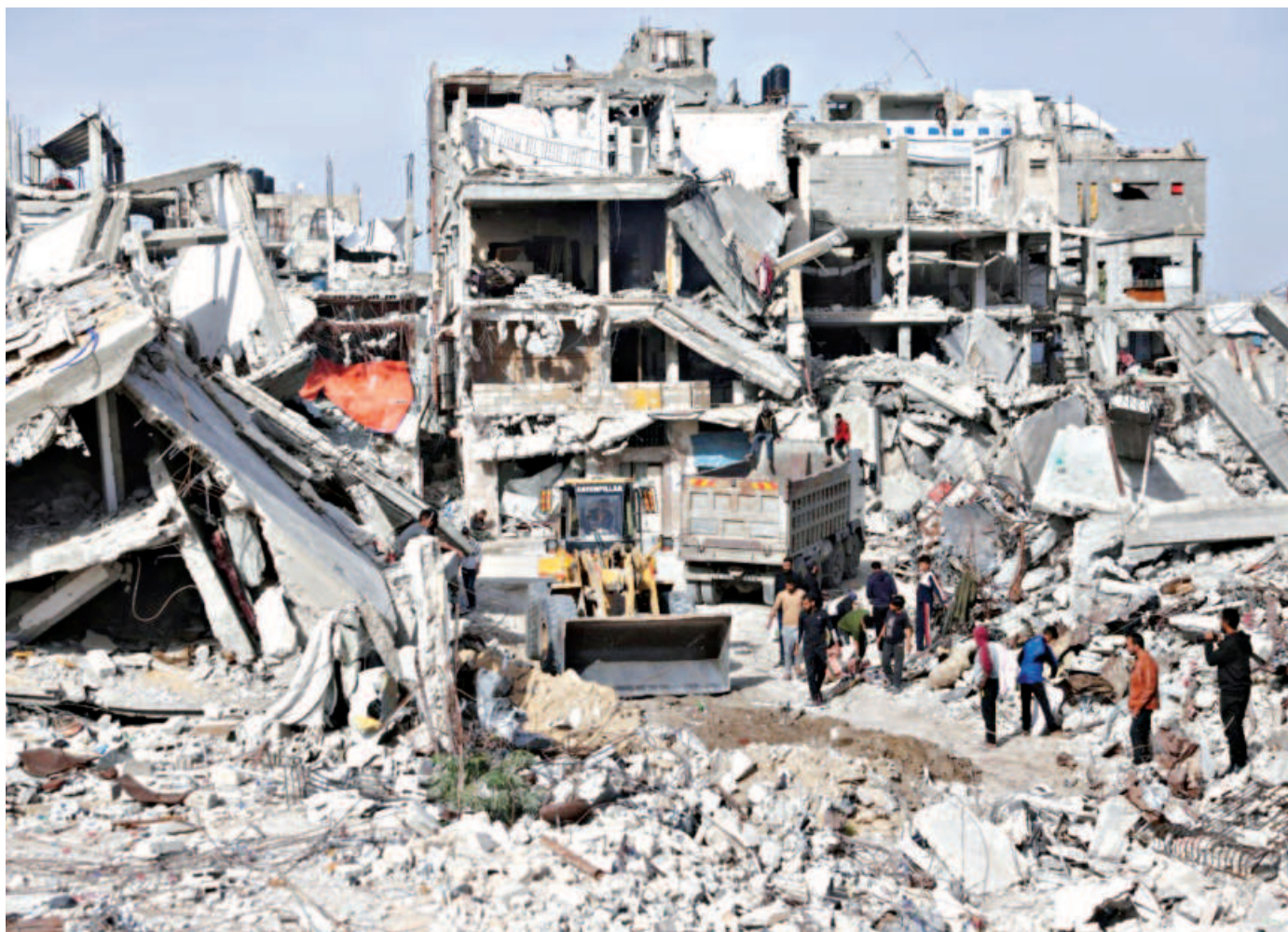
A Palestinian worker involved in a rubble management project maneuvers a digger to shift debris of destroyed buildings and houses in Khan Yunis in the southern Gaza Strip yesterday.
