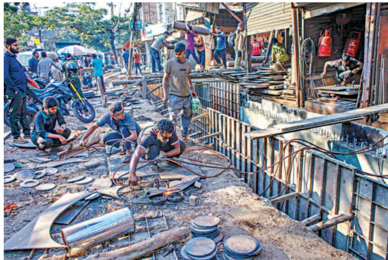
Labourers work with metal items without any safety gear, occupying a large section of the road in the capital's Dholaikhal area and putting themselves and pedestrians at risk. The situation is made worse by ongoing road development work, which further narrows the space for safe movement. The photo was taken yesterday.
