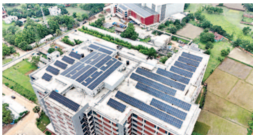
Drugmaker Renata PLC has installed rooftop solar panels at its Bhaluka site in Mymensingh to promote sustainability and reduce the environmental impact of its pharmaceutical operations. PHOTO: RENATA
