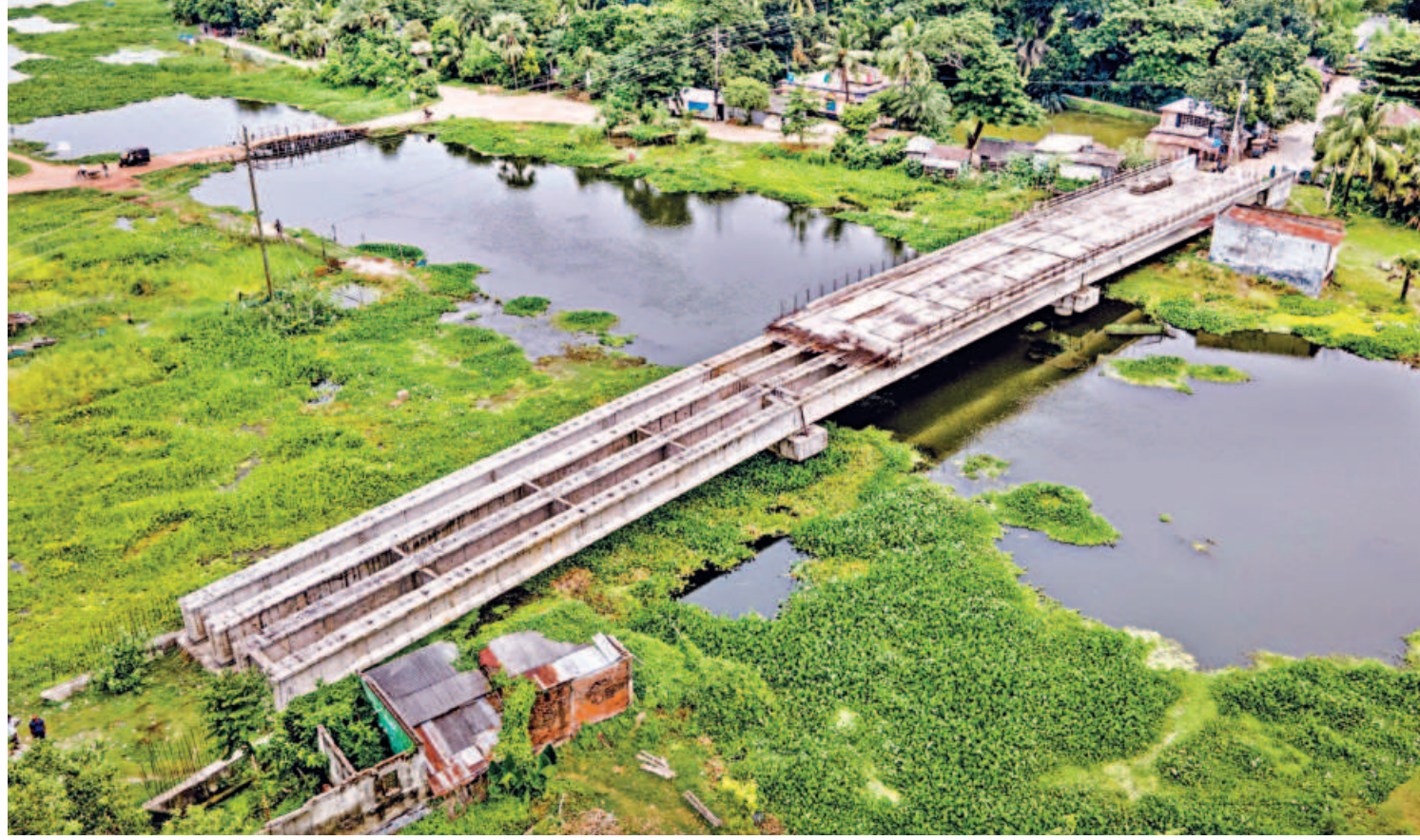
Construction of the Tekarghat bridge in Jessore's Abhaynagar has been halted for a long time, affecting the people of Abhaynagar and Manirampur upazilas. The work over the Teka river began in 2021 and was scheduled to finish by 2023. Locals now have to cross the river using a wooden bridge, top left.
