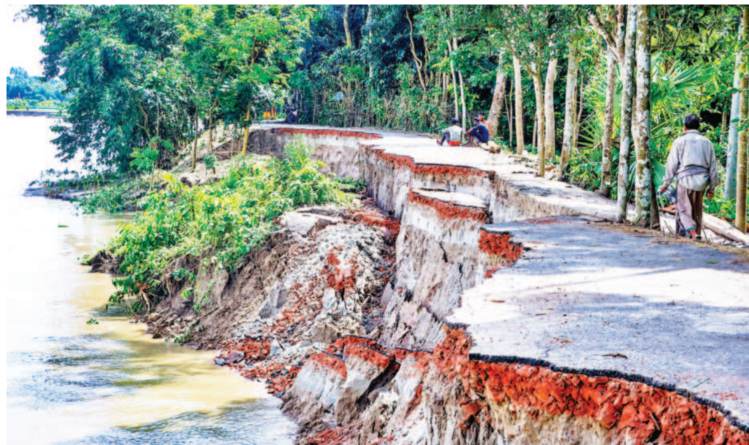
A large portion of a road in Chachoi village of Narail's Lohagara upazila has collapsed under pressure from the strong currents of the Madhumati River. Locals claimed continuous river erosion is also washing away cropland in the absence of a permanent embankment. The authorities concerned have yet to take any preventive measures. The photo was taken yesterday.
