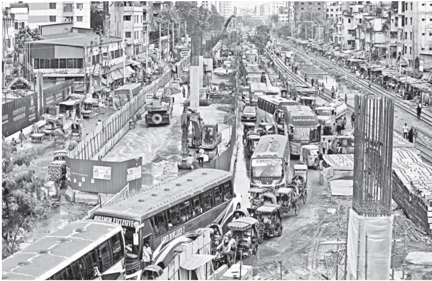
Scores of passenger buses, cars, and CNG-run autorickshaws remain stuck on a section of the road next to the under-construction Dhaka Elevated Expressway yesterday. Due to the construction work from Malibagh intersection to Khilgaon, the roadway has narrowed, causing severe traffic congestion in the area.
