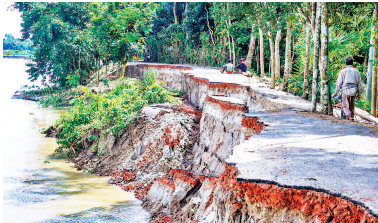
A large portion of a road in Chachoi village of Narail's Lohagara upazila has collapsed under pressure from the strong currents of the Madhumati River. Locals claimed continuous river erosion is also washing away cropland in the absence of a permanent embankment. The authorities concerned have yet to take any preventive measures. The photo was taken yesterday.
