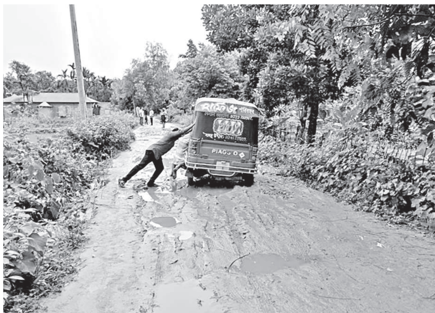
A CNG-run autorickshaw driver tries to push his vehicle out of a muddy pothole. This 1.5-kilometre stretch of Kalenga Road in Habiganj's Chunarughat upazila has fallen into disrepair, breaking apart whenever it rains and turning potholes into pools of mud and water.
