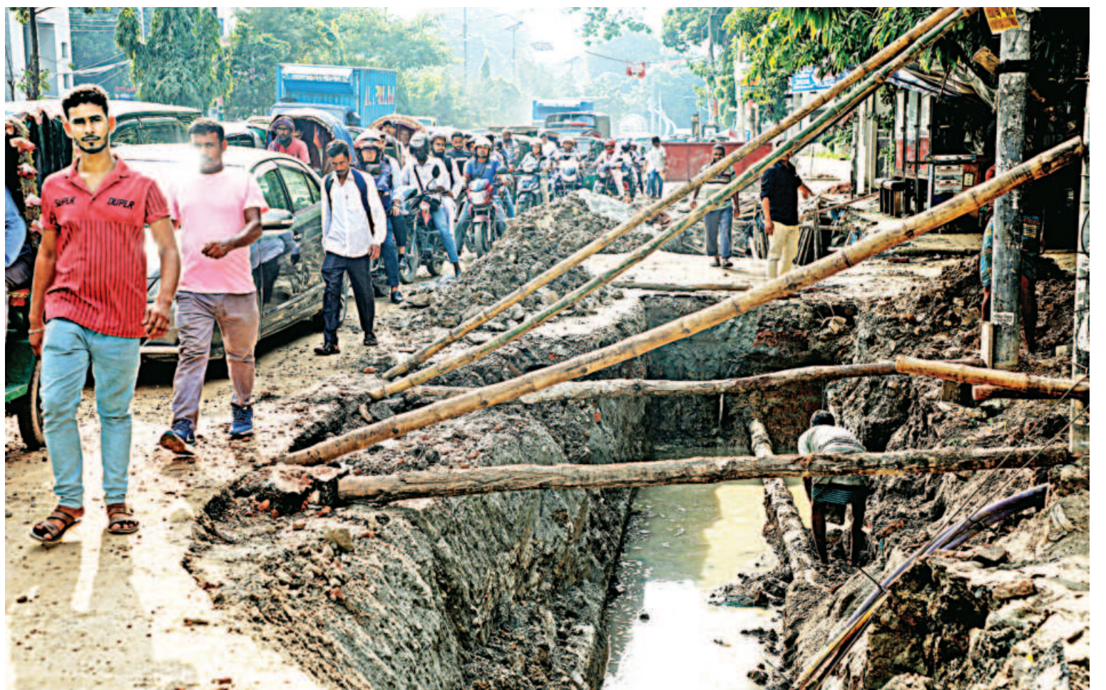
Dhaka South City Corporation carrying out drainage work without any safety barriers or warning signs in Kakrail, right next to Willes Little Flower School and College. This poses a risk of major accidents for vehicles and pedestrians passing through the area daily. The photo was taken yesterday.
