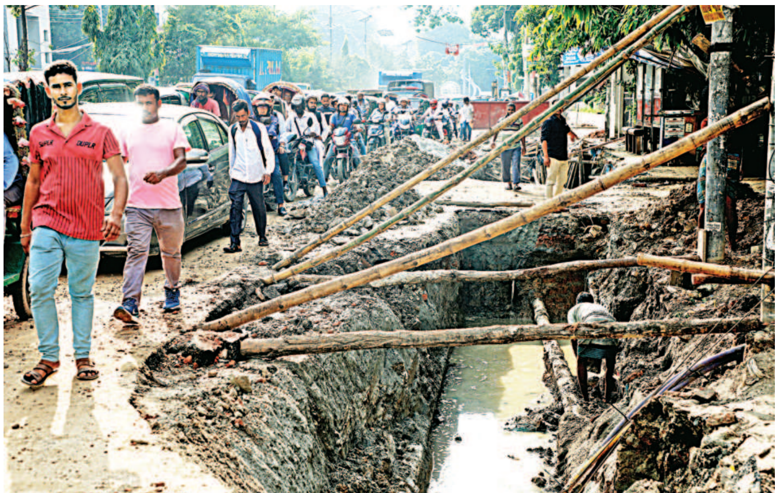
Dhaka South City Corporation carrying out drainage work without any safety barriers or warning signs in Kakrail, right next to Willes Little Flower School and College. This poses a risk of major accidents for vehicles and pedestrians passing through the area daily. The photo was taken yesterday.
