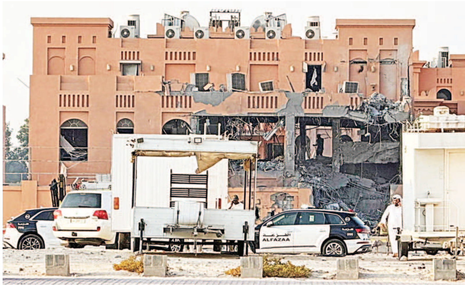
A building in Doha, Qatar, damaged in an Israeli strike, which Israel said was aimed at Hamas leaders, is pictured yesterday.
