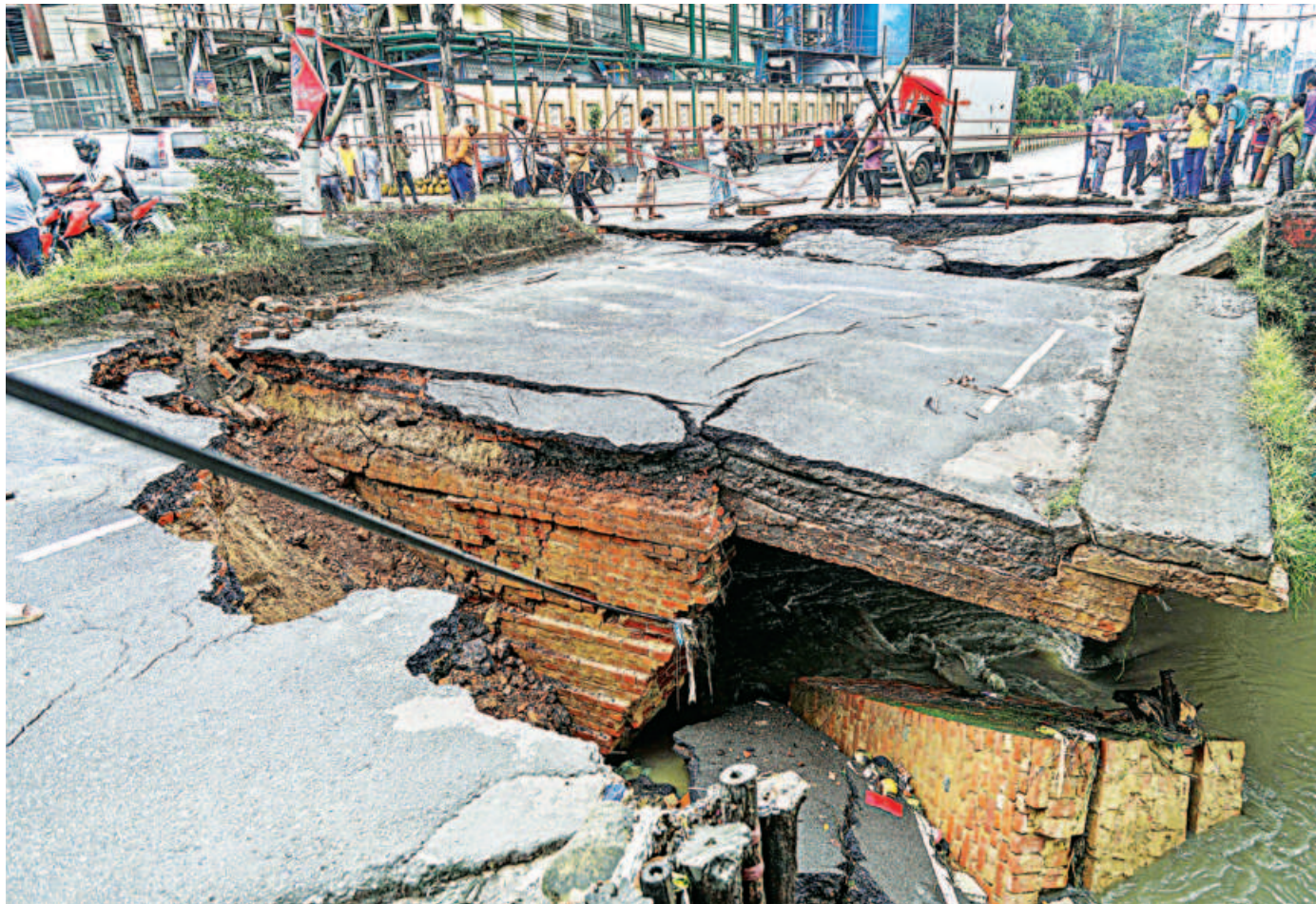
Heavy overnight rain on Wednesday caused the collapse of a section of the bridge over the Shital Jharna Canal in the Starship area on Gate No-2 Oxygen Road in Chattogram city, halting all traffic on one side. The photo was taken yesterday morning.
