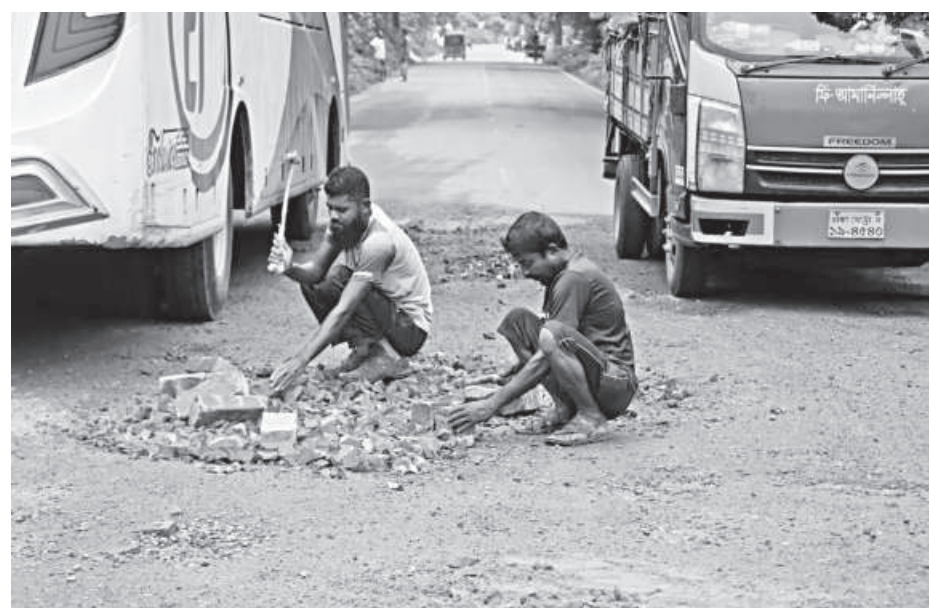
Workers of the Roads and Highways Department repair damaged portions of the Barishal-Kuakata highway. Following heavy rainfall last week, potholes have developed along the route, leaving it in a hazardous state. The photo was taken in Jhalakathi's Jurkathi area yesterday.
