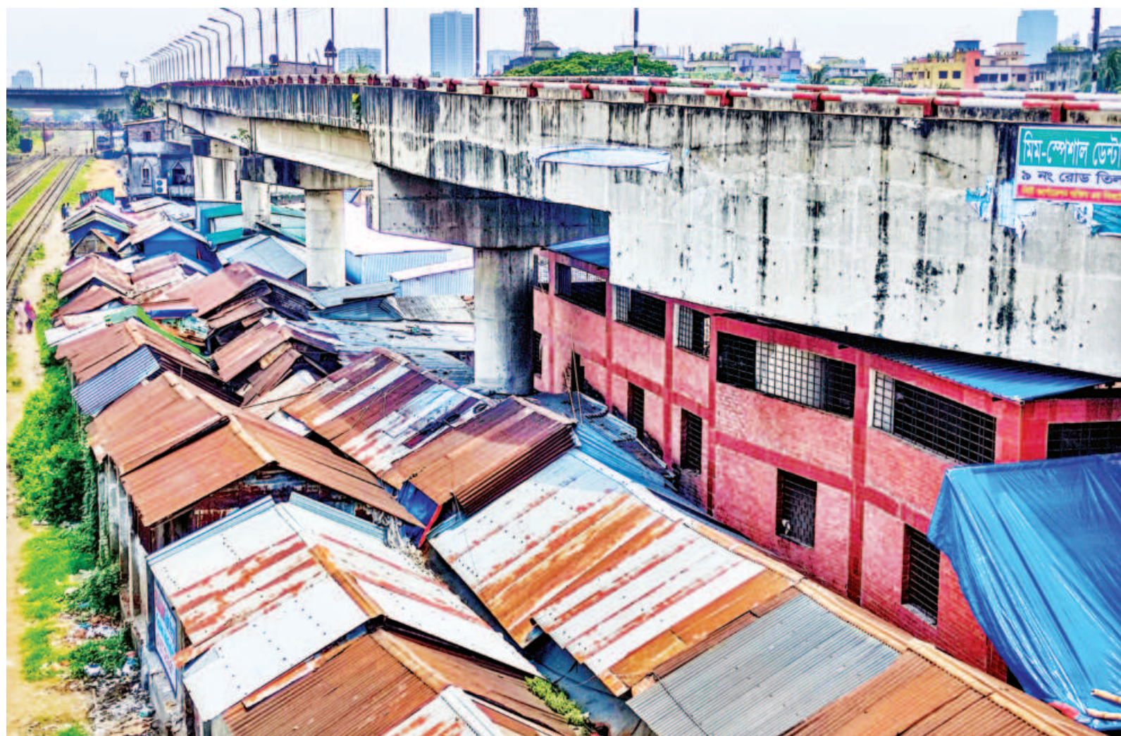
An illegal kitchen market has been set up on Bangladesh Railway land under the Khilgaon flyover, with rows of makeshift tin-roofed shops standing dangerously close to the railway tracks. The photo was taken yesterday.
