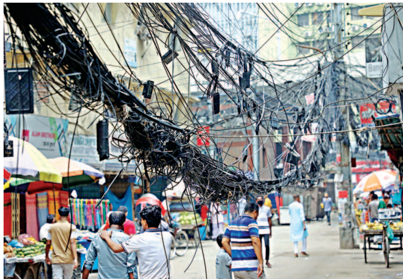
Pedestrians walk beneath a tangle of hanging cables, posing the risk of accidents at any moment. The photo was taken on Toyneeb Circular Road in the capital's Motijheel area recently.
