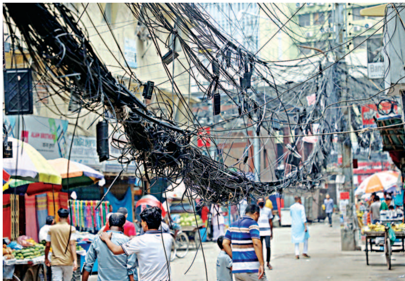
Pedestrians walk beneath a tangle of hanging cables, posing the risk of accidents at any moment. The photo was taken on Toyneeb Circular Road in the capital's Motijheel area recently.
